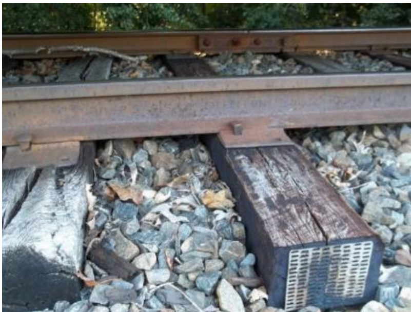
Figure 5-1 - Existing track structure with 100PS rail, single shoulder tie plates, timber ties and ballast
