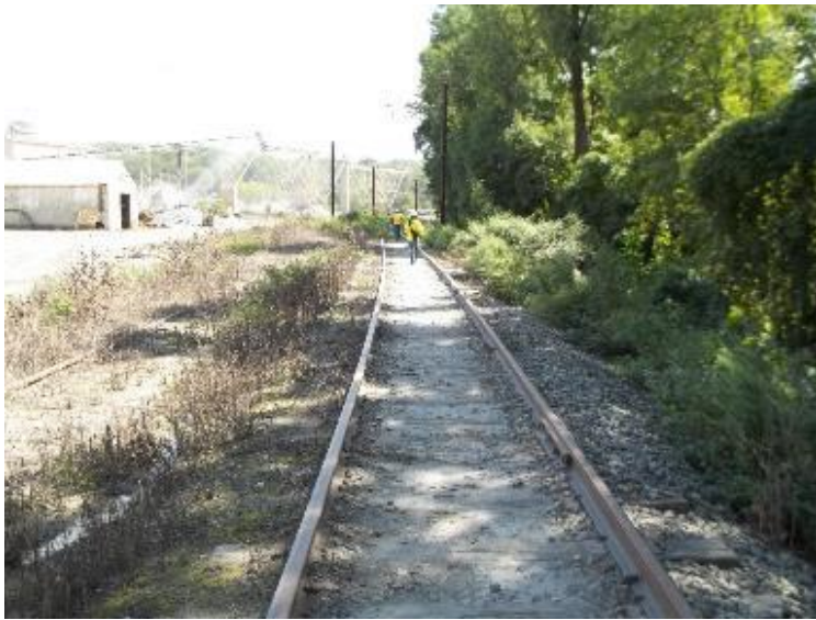
Figure 5-2 - Fouled ballast near quarry in Glen Mills
