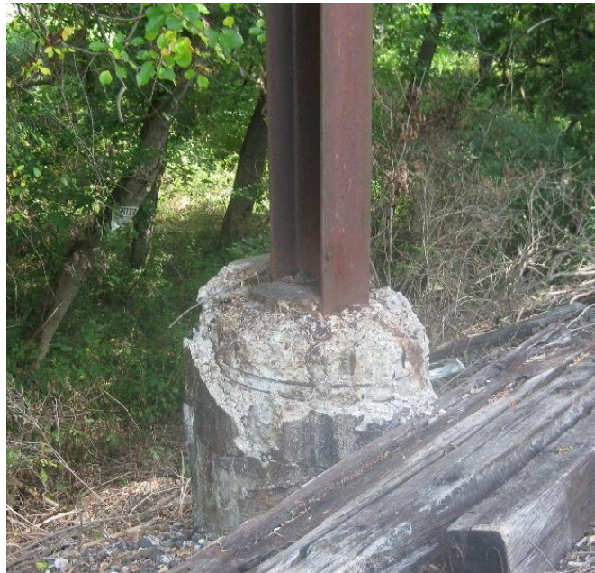
Figure 7-6 - Deteriorated catenary pole foundation
