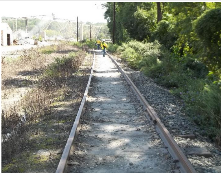
Figure 7-5 - Fouled ballast near quarry
