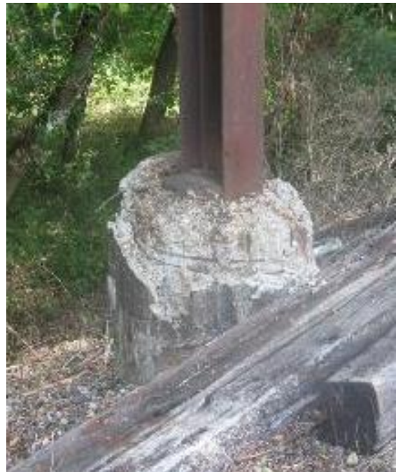
Figure 5-3 - Typical OCS Foundation with Exposed Rebar
